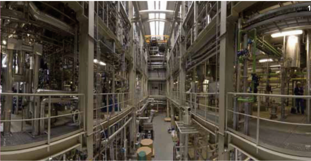
1 Polymer synthesis pilot plant in the pilot plant center.
